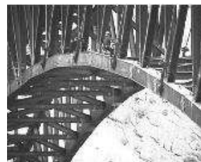
Fig. 23.7 Karun-3 steel arch.
