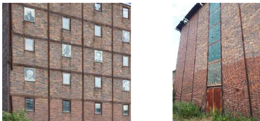
Fig. 7. Outer steel skeleton with corrosion damage
