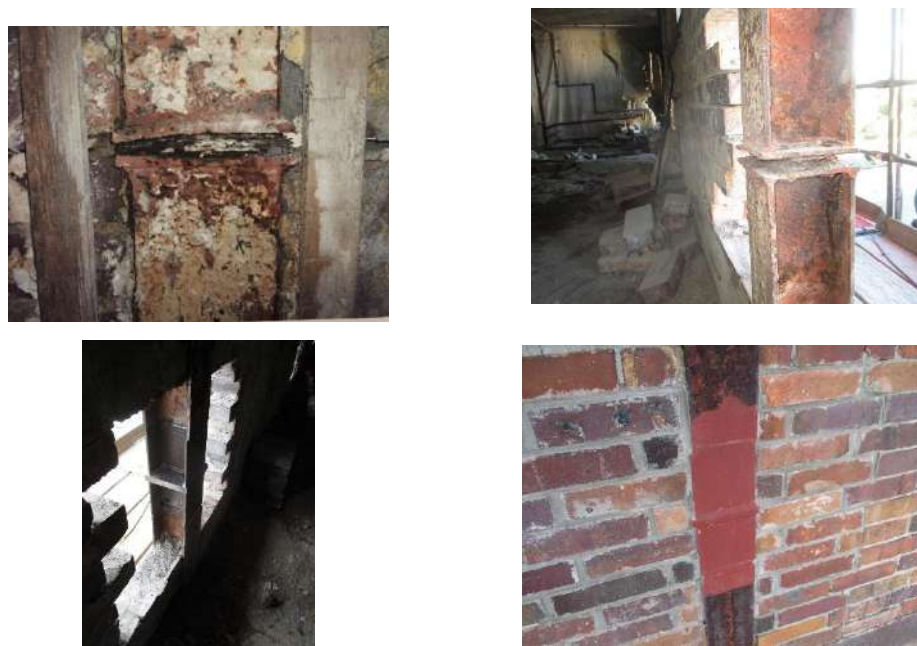
Fig. 8. Column in the building with corrosion damage and its rehabilitation
