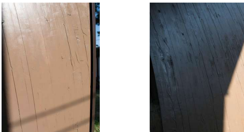
Fig. 4. Degradation of the main girders
