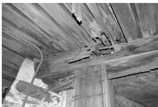
Fig. 19. Deteriorated girder and joists within a casemate.
