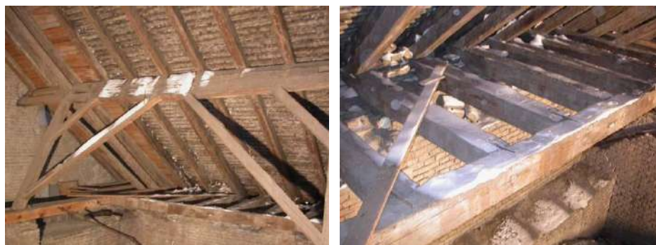
Fig. 13. Snow drifts on the roof structure as a consequence of roof cladding and battens damages
