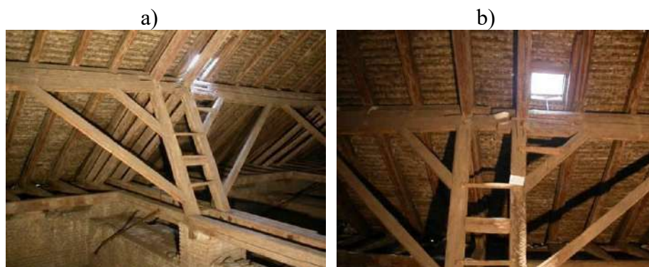
Fig. 16. Crack in the horizontal beam (a) and element fracture between trusses (b)
