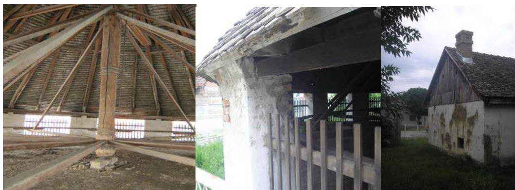
Fig. 2. Photos of damage pillar „popa, short walls of baked bricks and walls of adobe bricks
