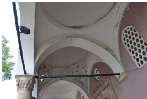
Fig. 7. Damages of the entrance arches
