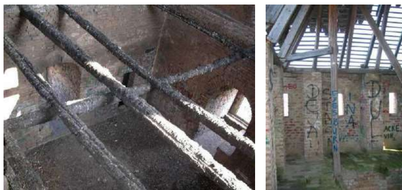
Fig. 4. Fire damaged timber floor joists and damages the roof structure
