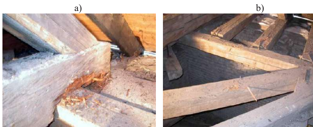
Fig. 14. Details of rot (a) and wormholes (b) in timber elements
