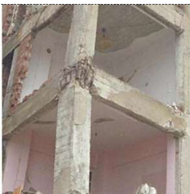
Fig. 5. Beam-column joint damage, Turkey, Koceli, 1999, after [17]
