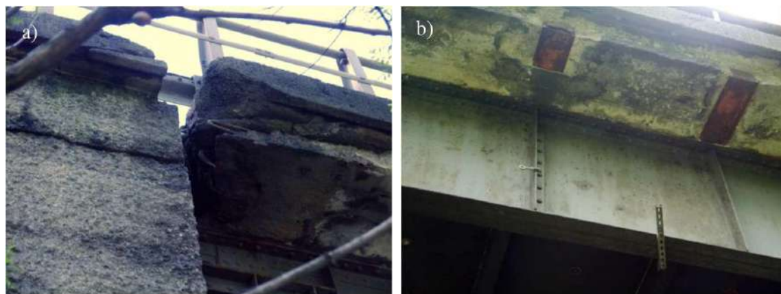
Fig. 9. Damages to the deck slab identified in its cantilever part, including: a) missing a piece of the deck in the vicinity of the abutment, b) corrosion of steel beams exposed to weather conditions after the concrete cover has fallen off.
