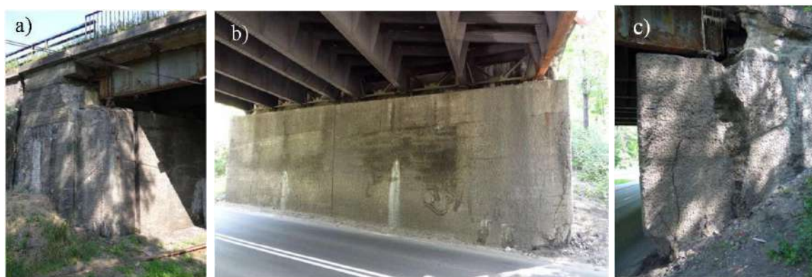
Fig. 10. Damages to the viaduct abutments (description in the text).
