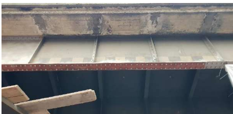
Fig. 18. The strengthening of the bottom flange used in the girder number 1.
