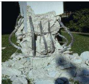
Fig. 1. Poor detail of transversal reinforcement
