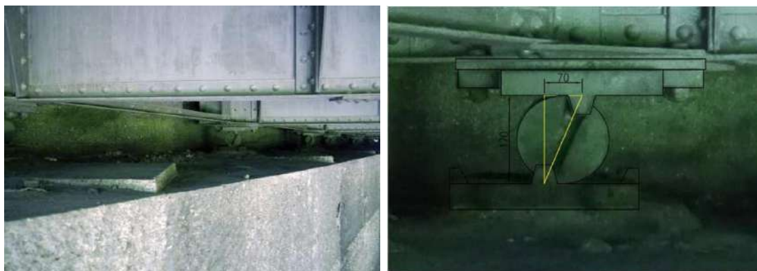
Fig. 12. The extreme deflections of the bearings observed at the abutment of the longer span.
