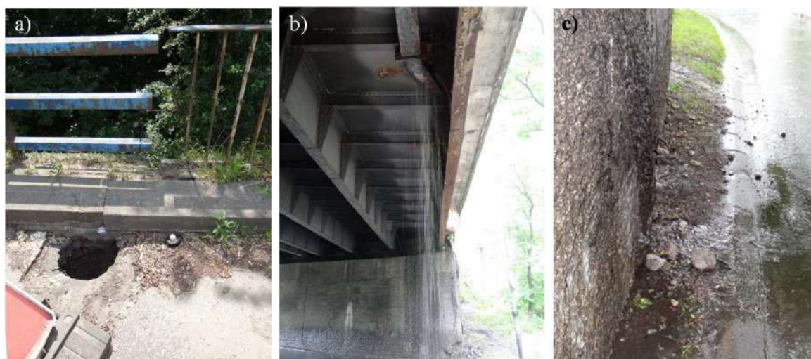
Fig. 7. Deficiencies in the viaduct drainage system, including: a) the lack of the protection of the drainage pipe, b) effects of a blocked drainage system, c) rainwater running down the abutment.
