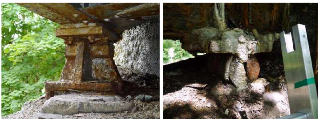
Fig. 11. Bearing corrosion inventoried under the outer girder.
